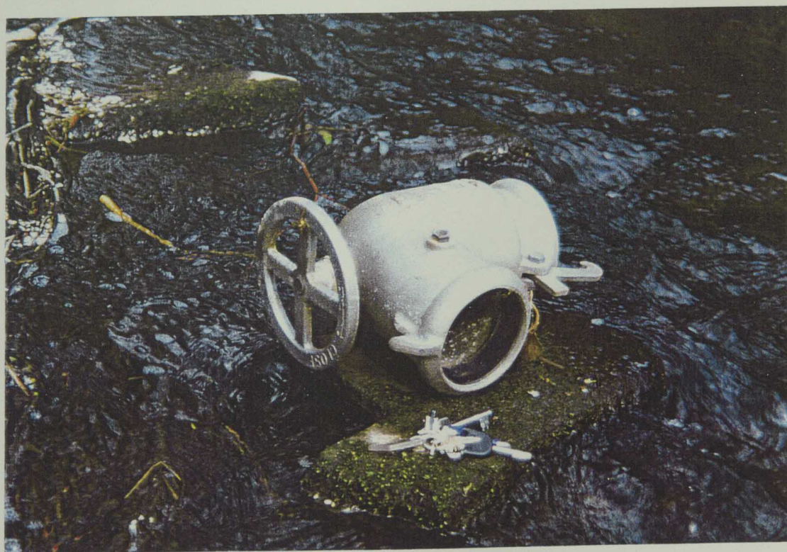
10. Photograph illustrating four inch abstraction pipe found in the gorge section of Canley Brook.
