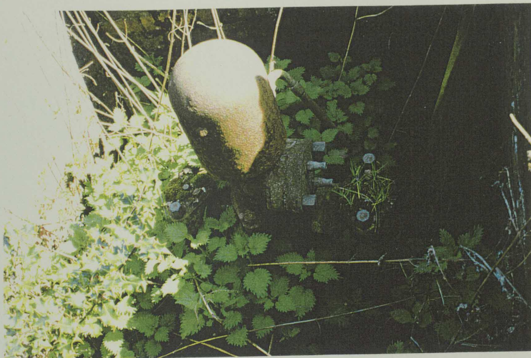
9. Photograph illustrating the pump machinery.
