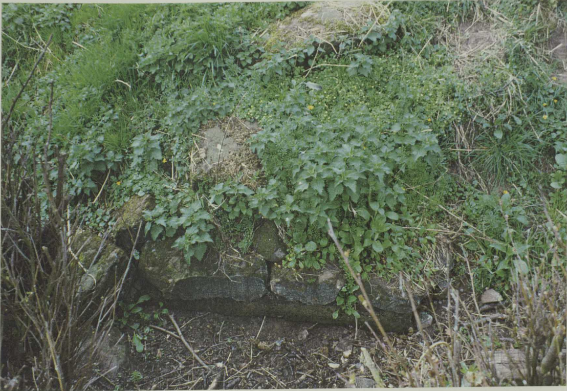
7. Photograph illustrating sandstone blocks in the tail race at site of earth dam.
