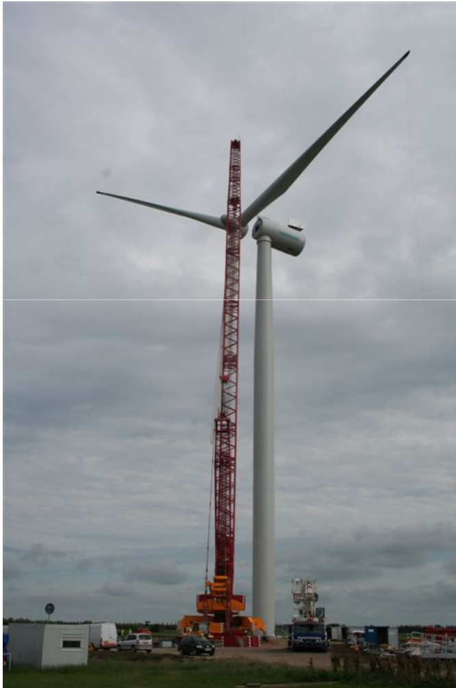
SWP 3.6DD on test at Tim (courtesy: Siemens Wind Power)
