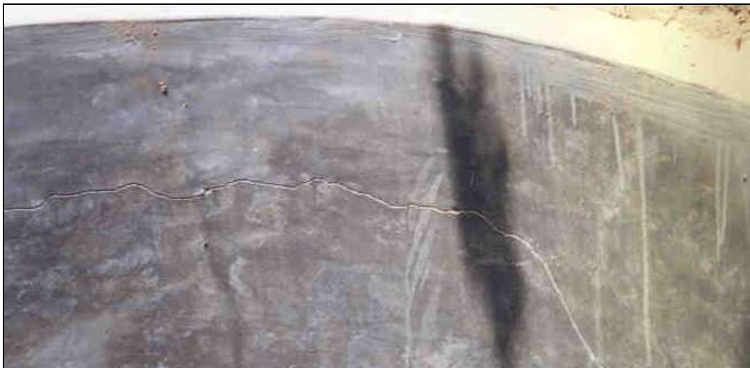
Figure 6.8: Horizontal cracks developed in an underground tank in Sri Lanka
