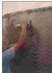
Application of the first layer of mortar on top of the wiring
