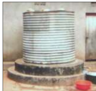
A corrugated steel tank in rural Uganda - note the concrete ring around the bottom repairing leaks [picture D. Rees]
