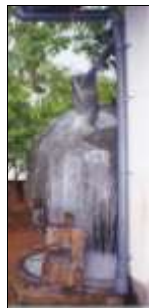
Simple downpipe first flush system in Sri Lanka (Picture:T. Ariyananda)
