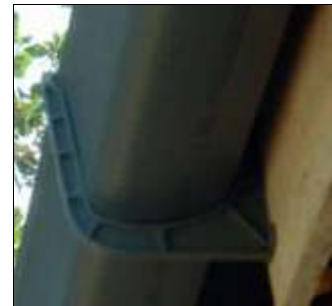
Plastic brackets mounting gutter to fascia board in Sri Lanka
