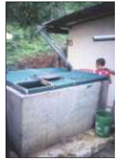
A plastered rectangular brick tank in rural Sri Lanka [Picture: D. Rees]
