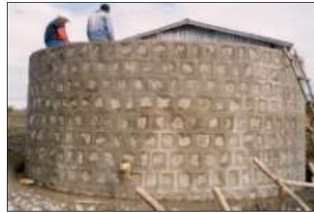
A communal masonry tank in Rural Ethiopia [Picture Water Action]
