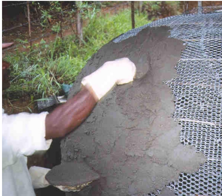
Figure 9.1: Applying mortar to the mesh and rebar formwork of the Pumpkin tank
