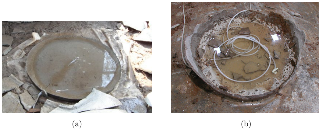
Figure 9.3: Base sections of two tanks after failure, showing (a) the joint debonding in the case of the tank produced with an internal mould and separate plastering of the base and walls, and (b) absence of such debonding in the case of the tank produced with an external mould and continuous plastering
