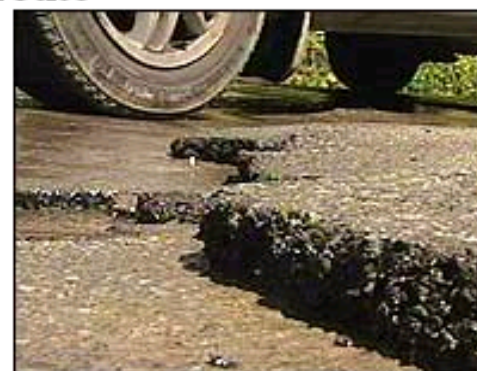
Damage to the county's roads is estimated to be £2.5m.
