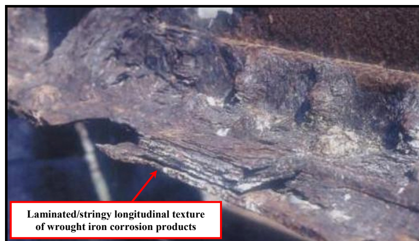
Figure 2-41 Excessive corrosion to a wrought iron construction beam 554
