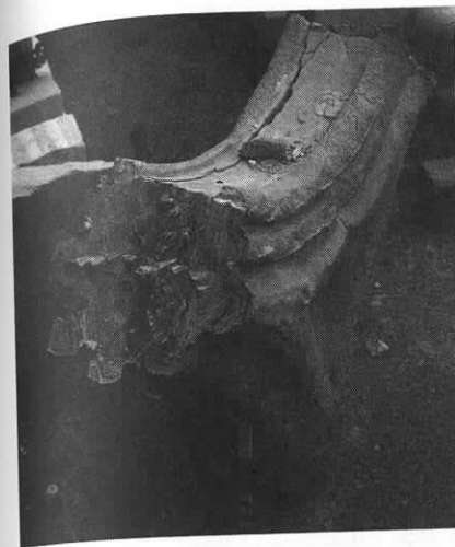
Figure 15.2 Salisbury Cathedral cloister; dismantled section of tracery showing lead joint in place (photo: author).
