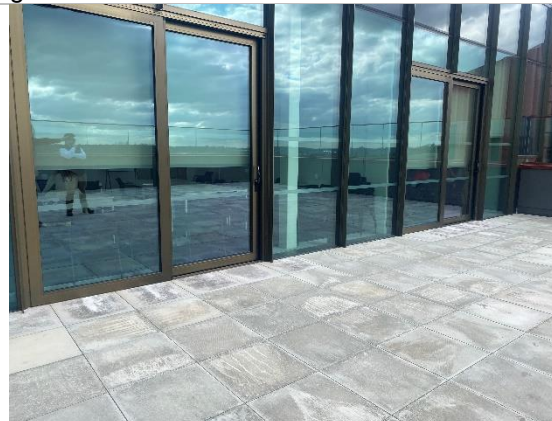
Double access doors that leads out from either classrooms or an open function space.
