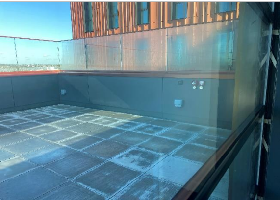
Fire detection point devices situated near main access door to balcony.
